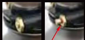
Red line on the pressure indicator
